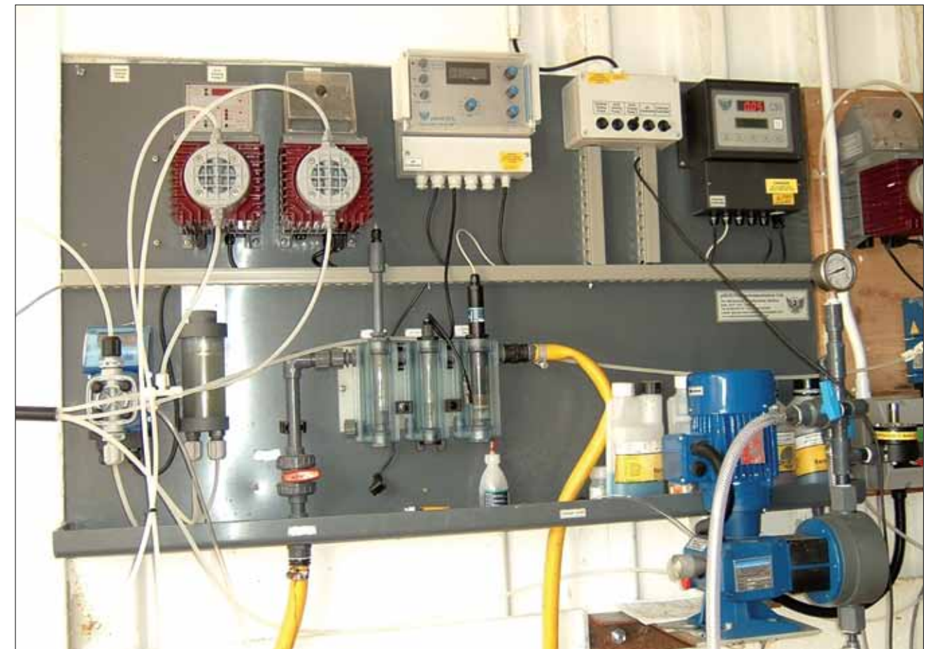
5 Chlorine injector used to kill bacteria in irrigation water
